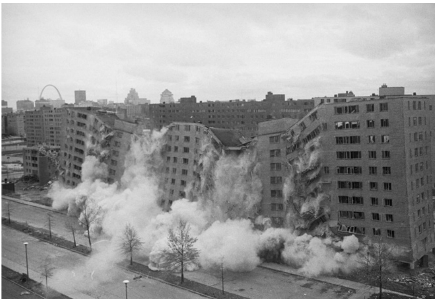
The demolition of the Pruitt-Igoe public housing complex in St. Louis, Missouri, in the 1970s marked the beginning of a national reconsideration of affordable housing production and finance. Credit: Bettmann/Getty Images.
