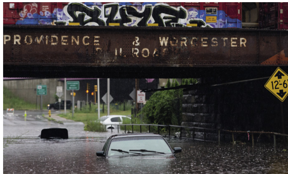
Cars navigate heavy flooding under an aging Providence & Worcester Railroad bridge in Worcester in July 2018. Credit: Matthew Healey
