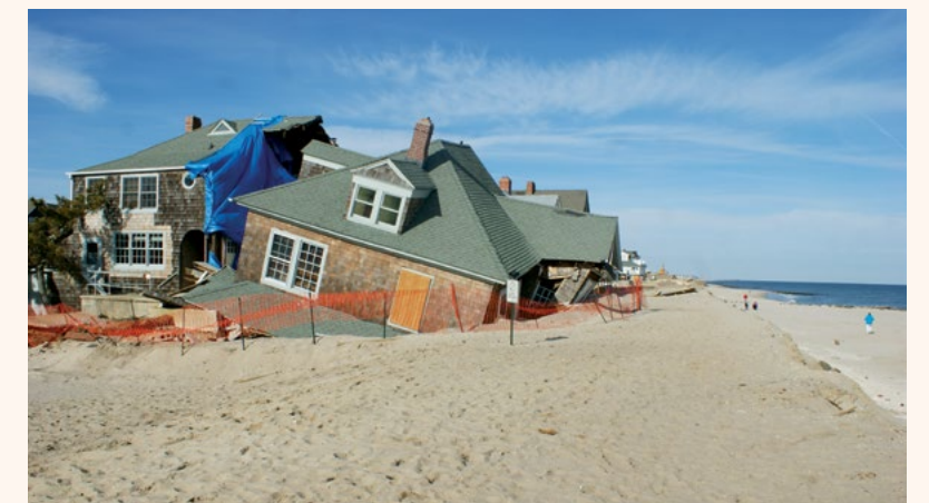
Hurricane Sandy damaged many homes along the New Jersey shore after making landfall there on October 29, 2012. Source: L. Johnson (2013).
